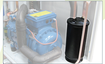
Suction Line Accumulators
