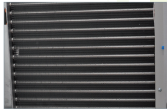
Efficient use of Condanser
